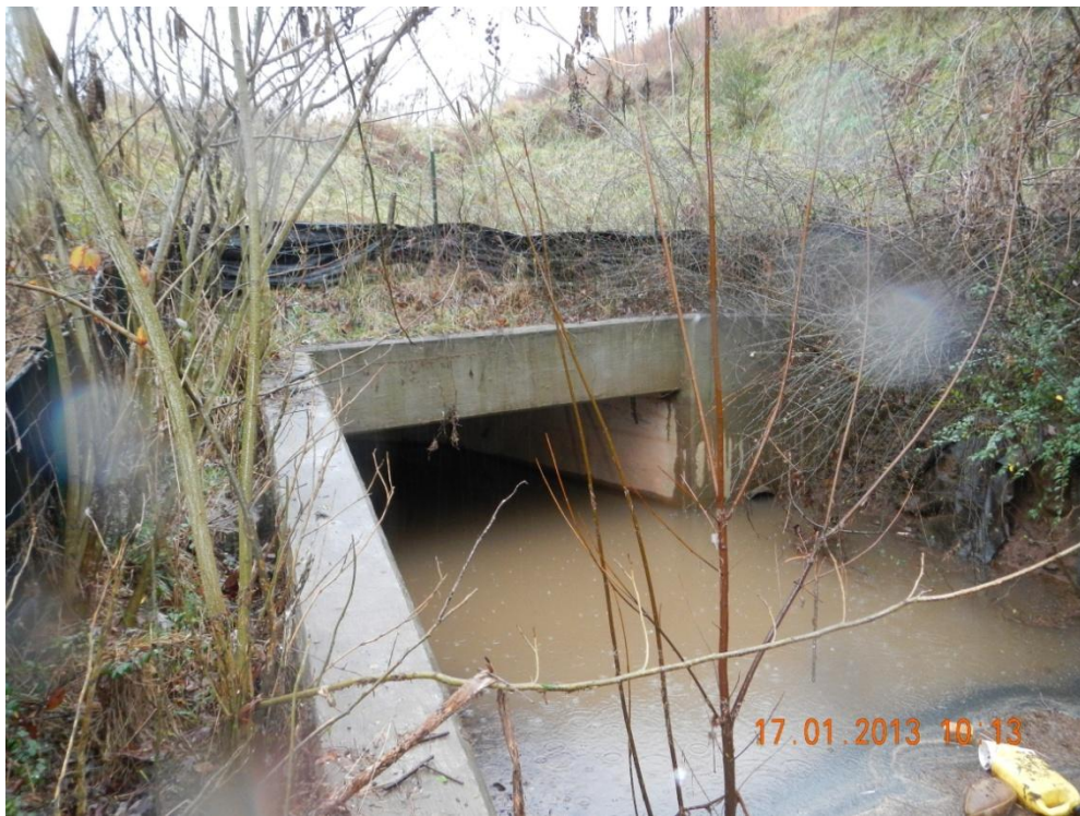
Photograph 6 – DSCN0017. N35.4323°, W-84.5858°. View of STR-3 (Gilbert Hollow Branch) facing upstream and east at the outlet of the existing structure near STA 97+00R.
