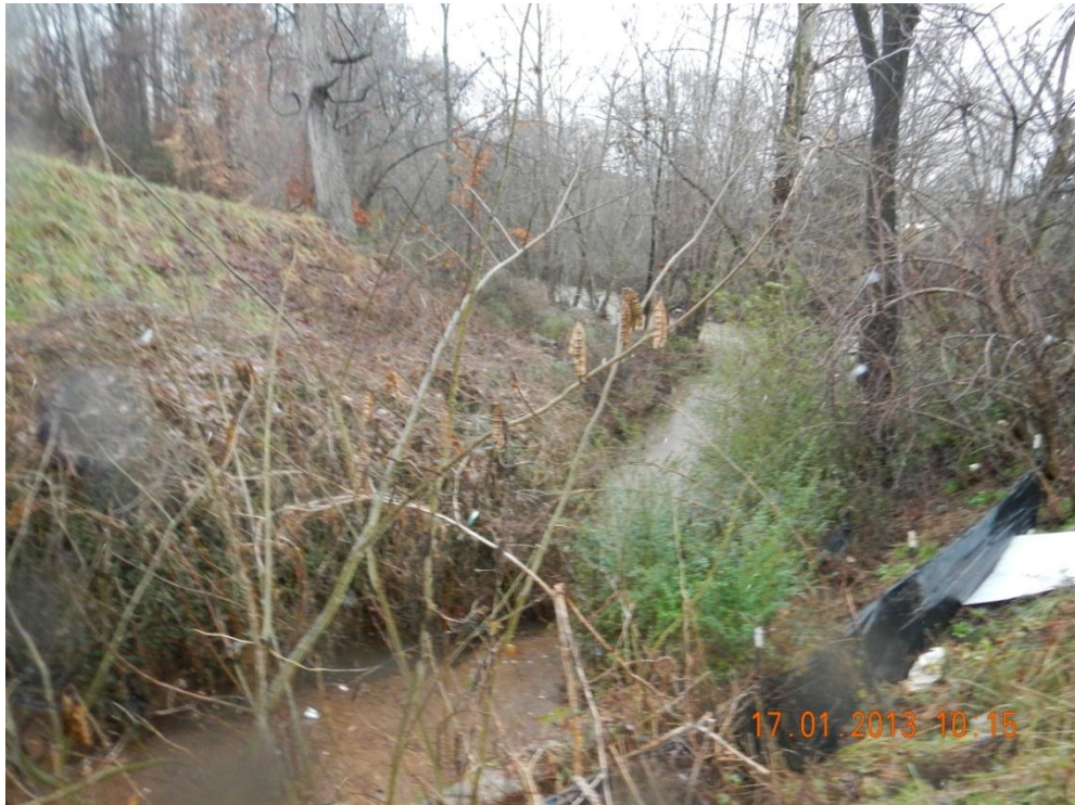
Photograph 7 – DSCN0019. N35.4323°, W-84.5858°. View of STR-3 (Gilbert Hollow Branch) facing downstream and west at outlet of existing structure near STA 97+00R.
