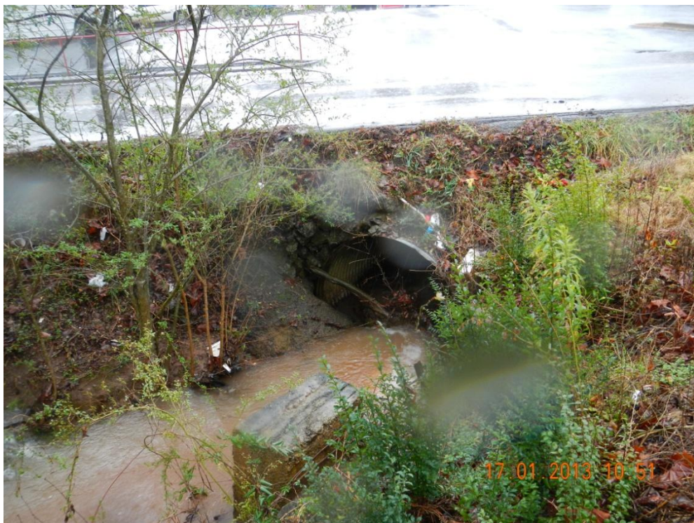
Photograph 8 – DSCN0025. N35.4314°, W-84.5838°. View of STR-3 (Gilbert Hollow Branch) facing downstream and west at inlet of existing structure beneath S. Jackson St. near STA 102+50L.
