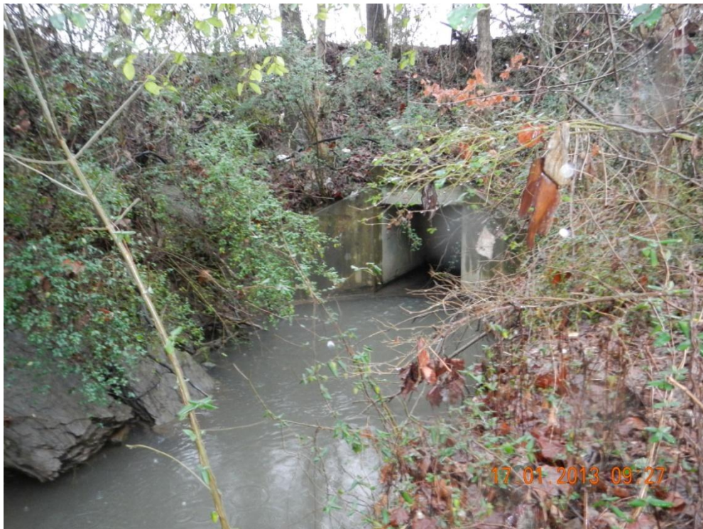
Photograph 4 – DSCN0007. N35.4380°, W-84.5896°. View of STR-2 facing upstream southwest at STA 73+00L.
