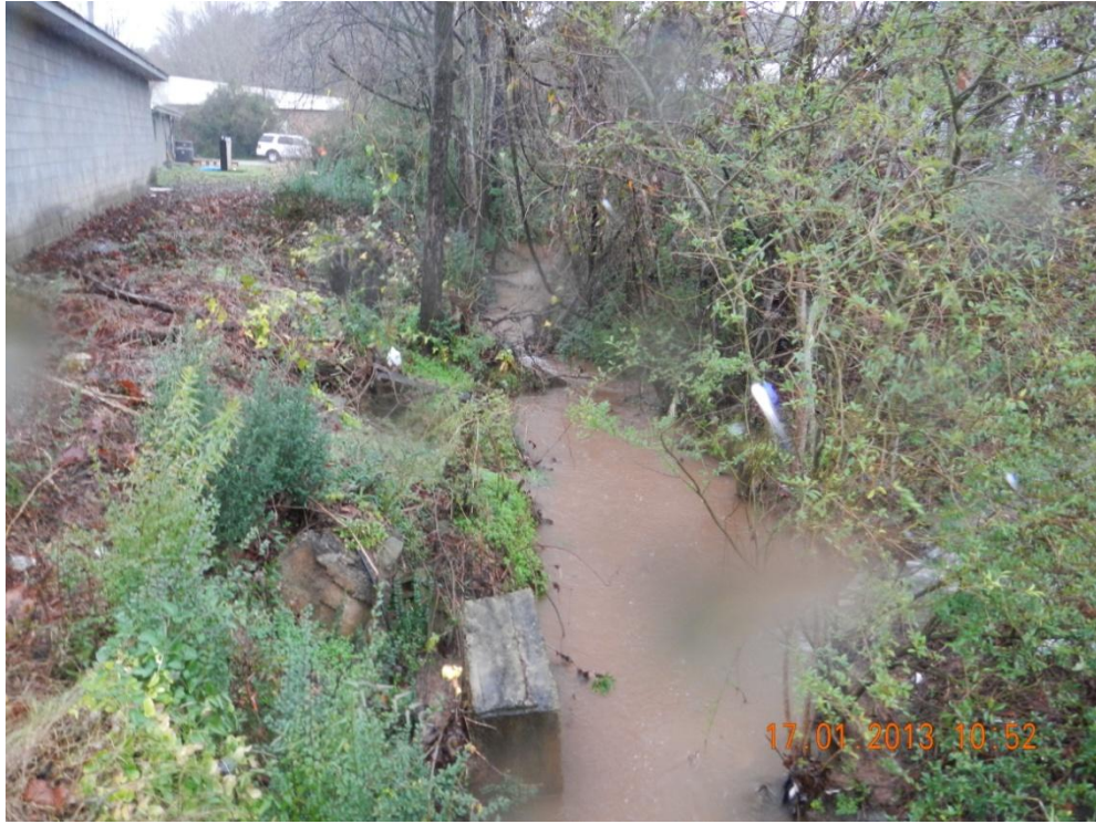
Photograph 9 - DSCN0026. N35.4314°, W-84.5838°. View of STR-3 (Gilbert Hollow Branch) facing upstream and east at inlet of existing structure beneath S. Jackson St. near STA 102+50L.
